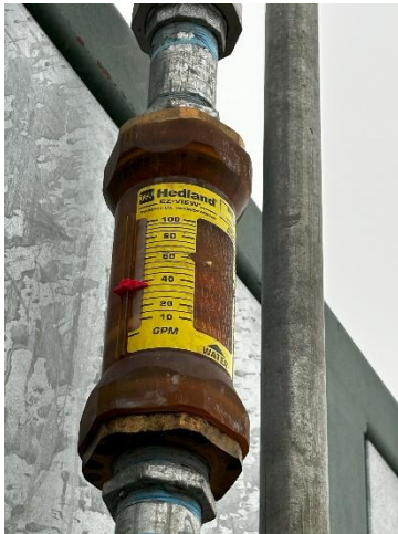
Figure 22: Heat recovery water flow meter.
