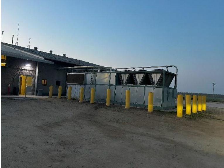
Figure 4: Hybrid chiller at Site-1.
