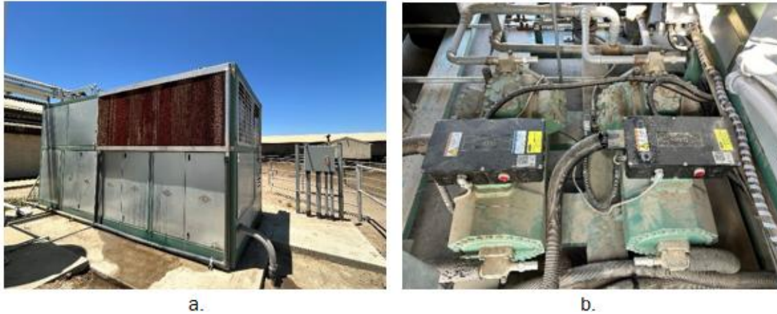
Figure 6: CO 2 chiller at Site-2 (a). CO 2 compressors (b).
