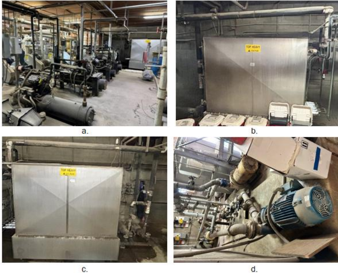
Figure 5: Westside and eastside chillers (a). westside evaporator (b). eastside evaporator (c). condenser water pumps (d).
